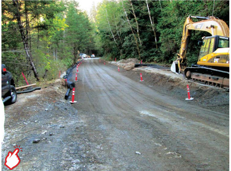
FIGURE 1 Construction of the Agness Road deep patch in Oregon in 2014. The second layer of geogrid is installed and covered with gravel.
