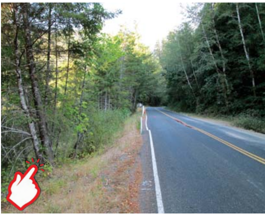
FIGURE 8a Agness Road site before deep-patch construction in September 2014.
