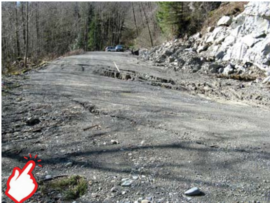
FIGURE 5a Before photograph in March 2015 of the MFSRR Milepost 10 deep patch.
